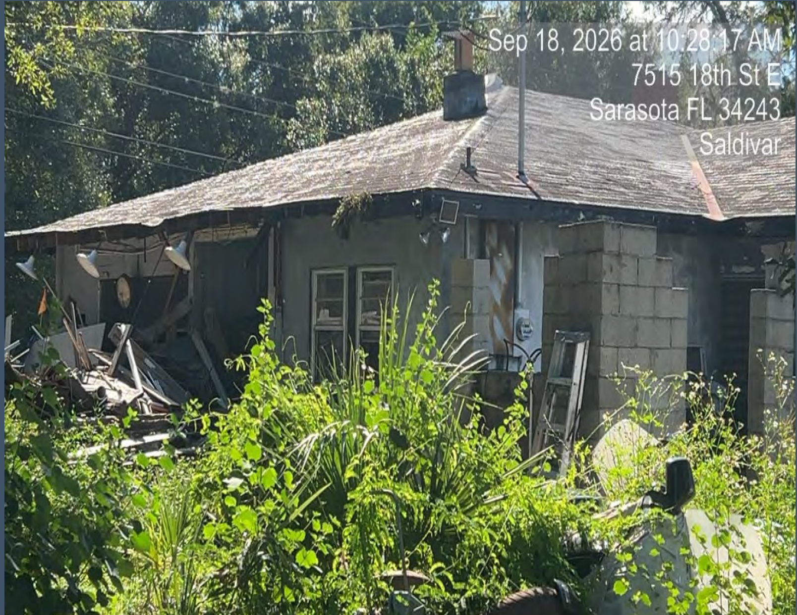
Picture depicts the roof with part of it collapsed and missing fascia.
