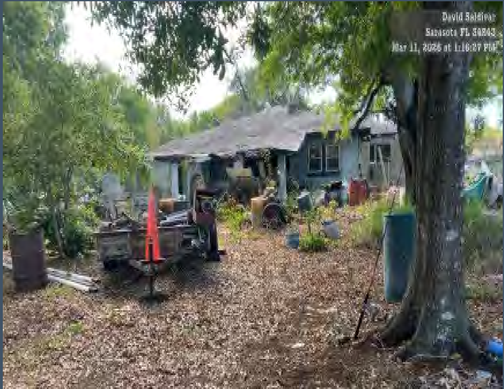
Photo depicts the roof in disrepair on the north side of the house.
